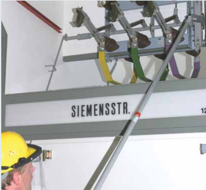
Switching a disconnector by means of an SCS switching stick
