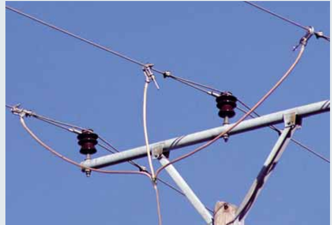
Phase screw clamps used on an overhead line
