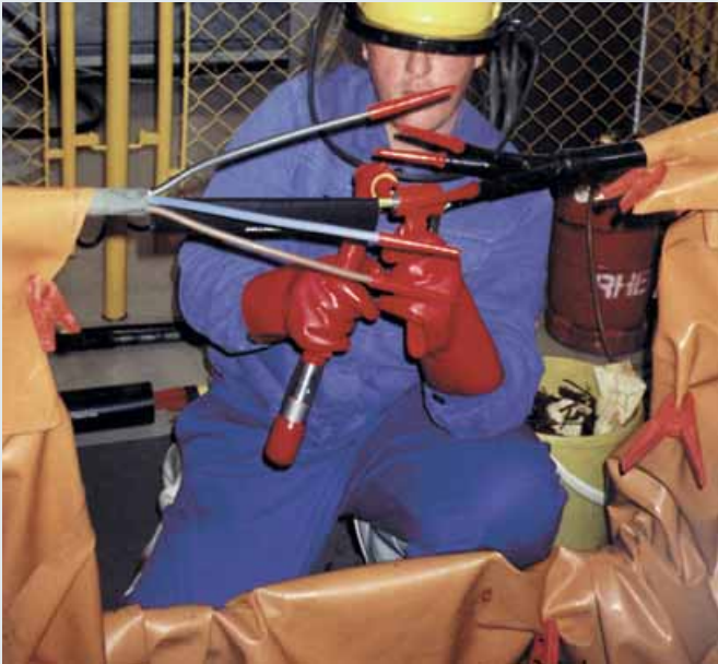
Covering live parts
