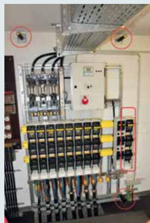
Figure 2: Fixed components for the mobile arc fault protection system
