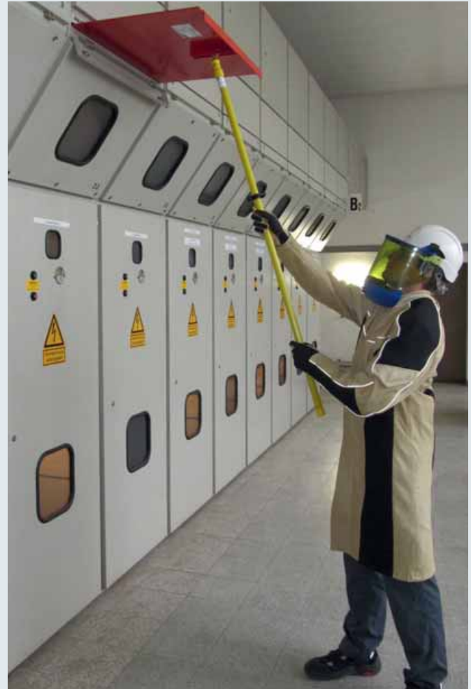
Inserting an insulating protective shutter (type A3) by means of an operating stick
