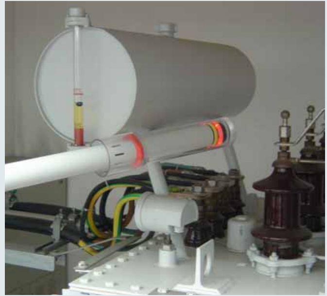
HSA 205 non-contact voltage detector with insulating cap used on a switchgear installation
