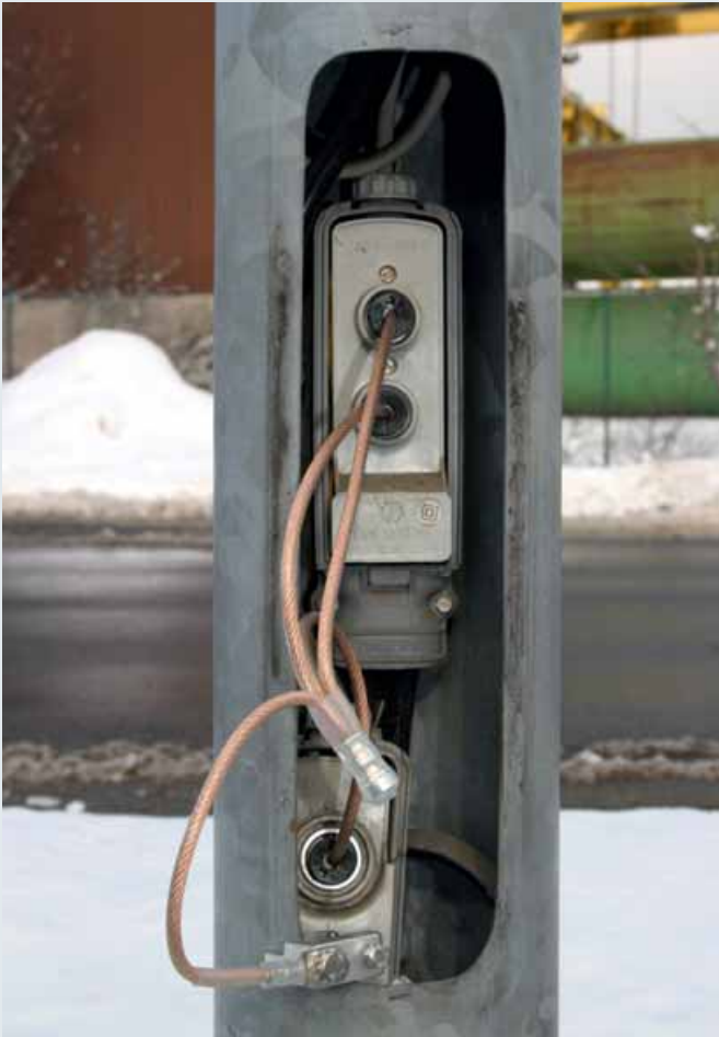
Earthing and short-circuiting device installed at a junction and fuse box of a street lighting mast
