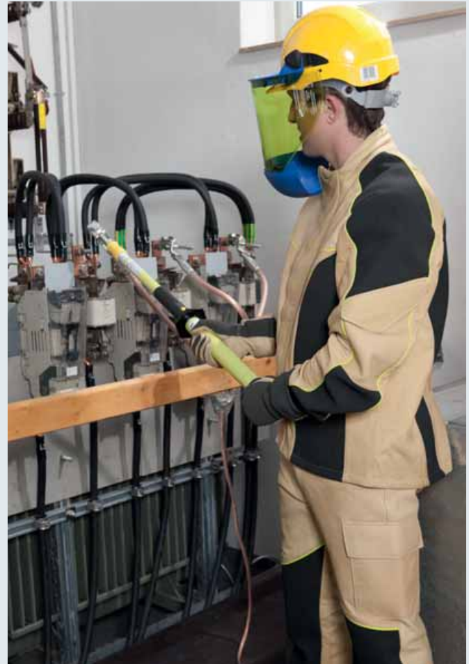
Attaching an earthing and short-circuiting device using adequate personal protective equipment
