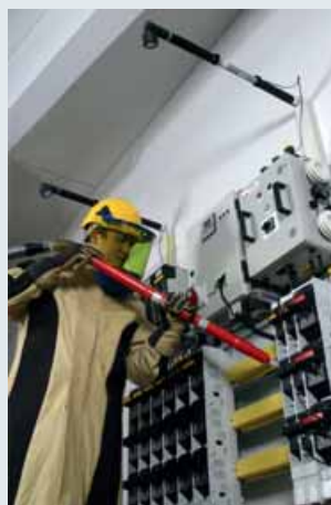
Figure 3: Work on an open switchgear installation using a mobile arc fault protection system
