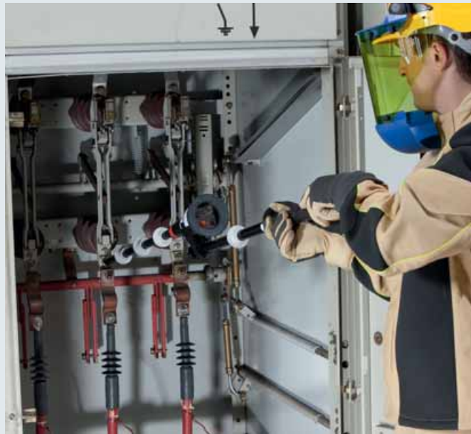
Single-pole PHV I phase comparator used in a switchgear installation
