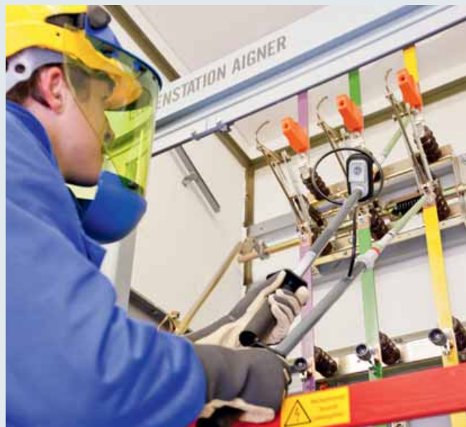
Two-pole PHV phase comparator with a pair of green test prods (15 ... 24 kV) used in a 20 kV switchgear installation
