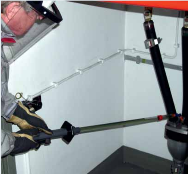
Refilling of hot HT mass under live conditions
