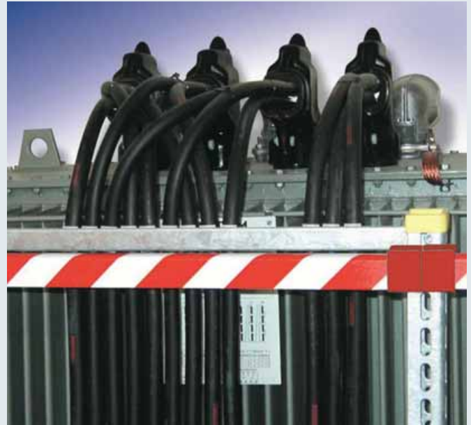
Barrier in a transformer station
