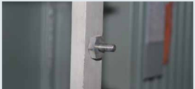
Bolted-type earth connector with M12 threaded pin on an earthed part of an installation
