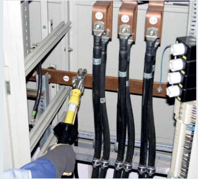
Attaching an earthing and short-circuiting device in a low-voltage switchgear installation using an earthing handle
