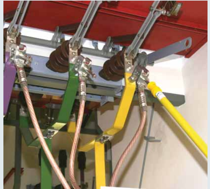
Earthing stick used for attaching an earthing and short-circuiting device to an installation
